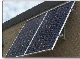
Wall Mount Solar Array
