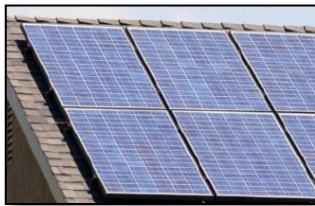
Roof Mount Solar Array
